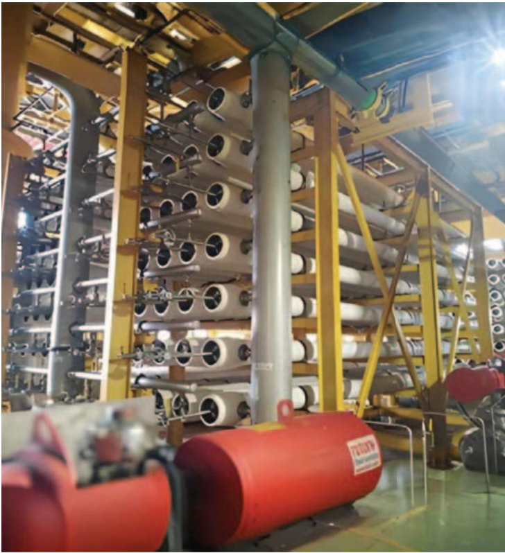
Sea Water Reverse Osmosis (SWRO)
