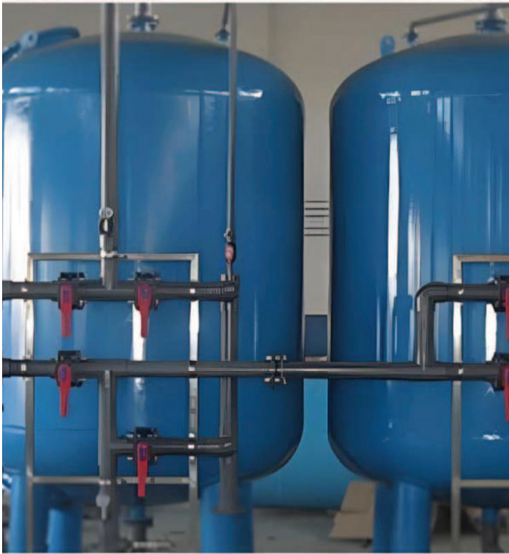
Pressure & Sand Filter
