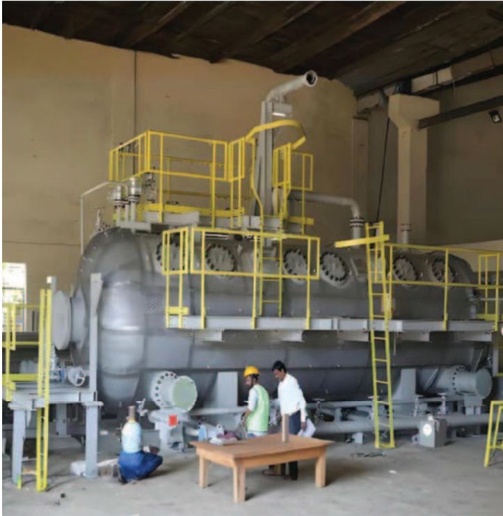
Induced Gas Flotation (IGF)
