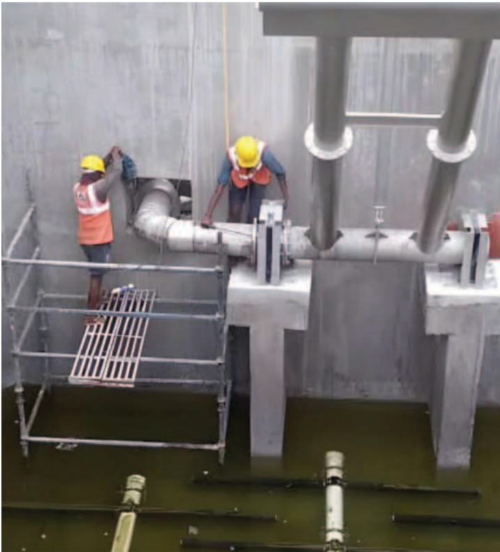
Sequential Batch Reactor (SBR)
